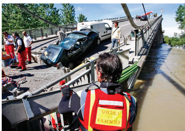
Figure 3 Piacenza, 30 April 2009. The collapse of one of the bridges across the Po' (photo: P Caridi, WordPress, available from http://peppecaridi2.wordpress.com/ ).
